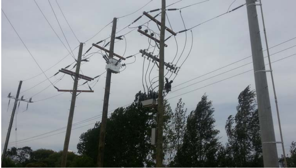
Recently Designed 33kV Private Line with ABS/Recloser/Metering Unit for HVC
