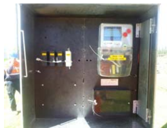
High Voltage Metering
