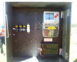
High Voltage Metering
