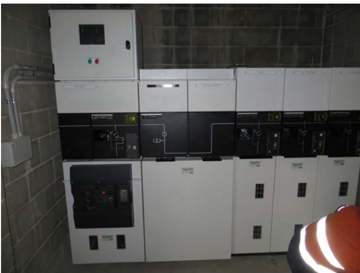
High Voltage Switchgear
